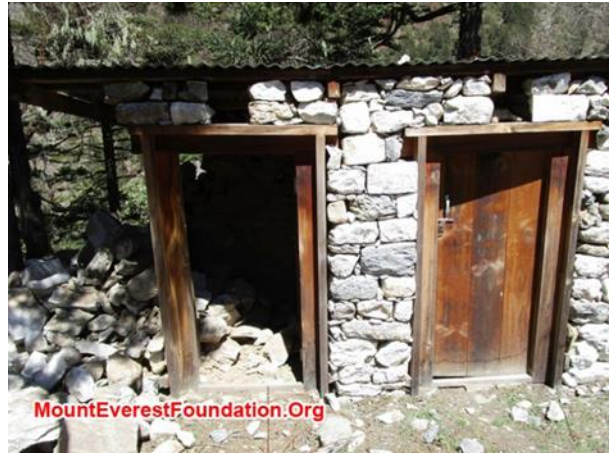
2015- left side with wall damage
